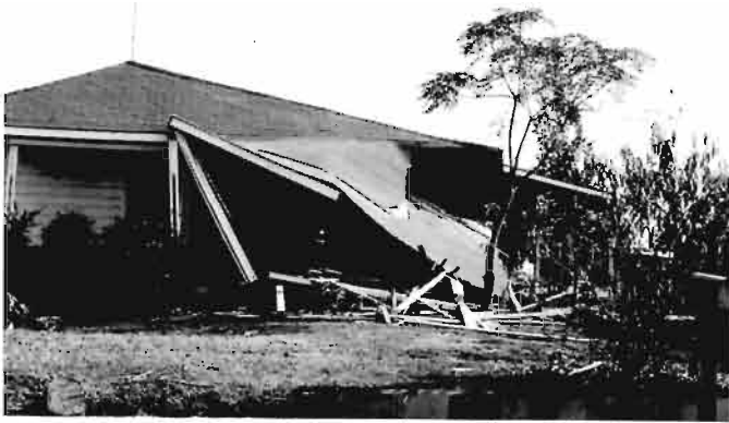
THE WRECKED HOME of Mrs. Aleyne Quinn. A bomb blasted all but one of the eight rooms of the house.
