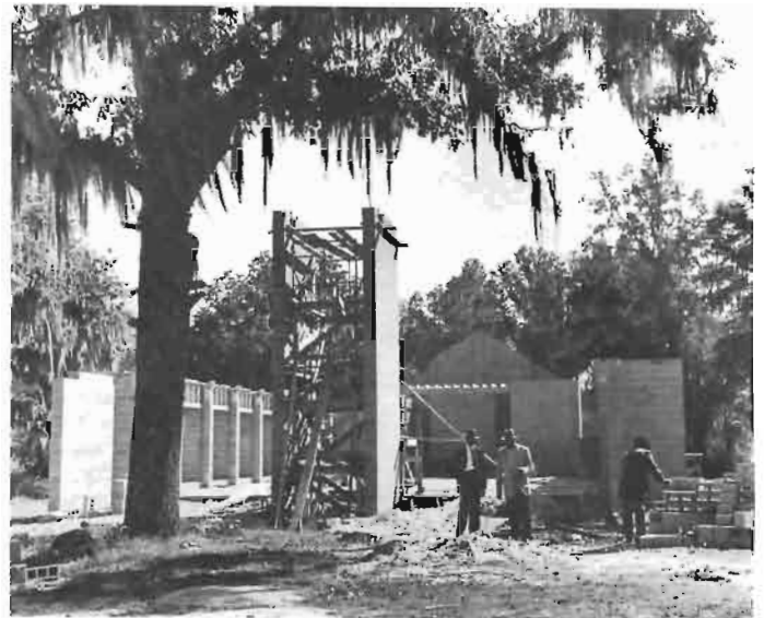
VANDALISM BEFORE COMPLETION—Although construction of churches is still going on, vandals already have tried to halt their completion. Thirty-foot pier like that shown above was yanked down recently during night at Mount Mary Church in Terrell County, Georgia.
